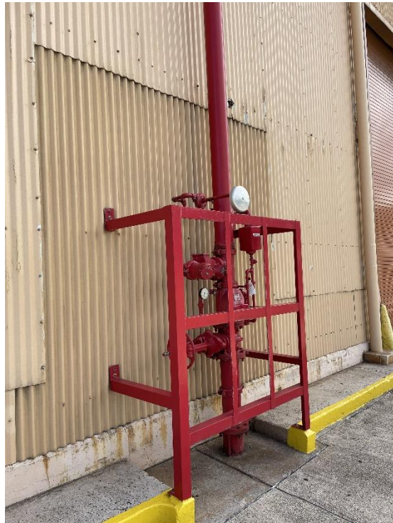
Photo 4: Example of new fire sprinkler system.
